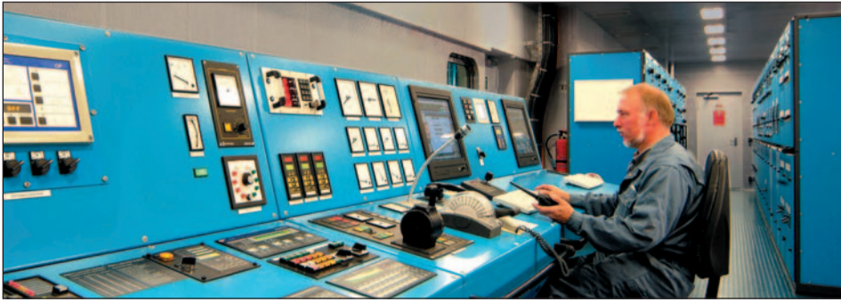
The Lyngso Marine 2200 Series automated integrated control system
